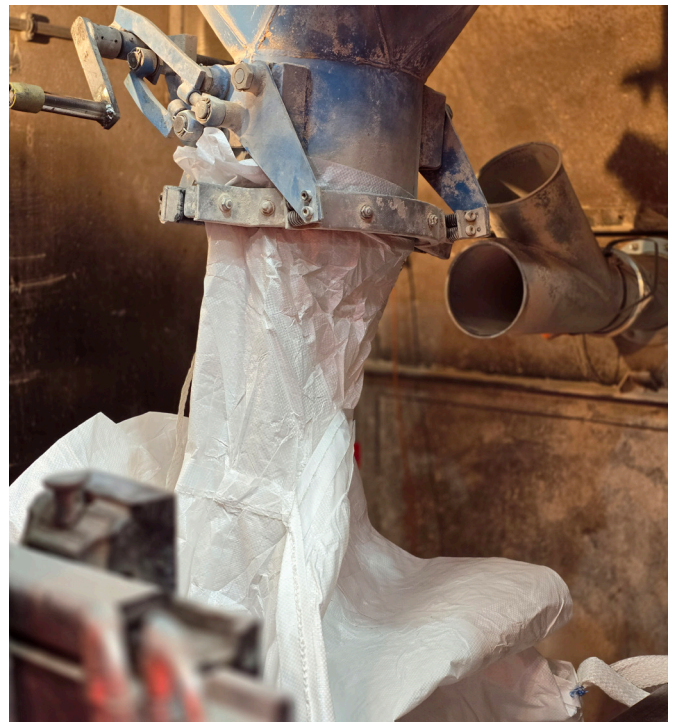
Ineffective clamp system used to hold bulk bags in place
