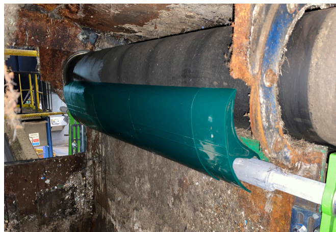
Starclean pre-cleaner installed on troublesome conveyor
